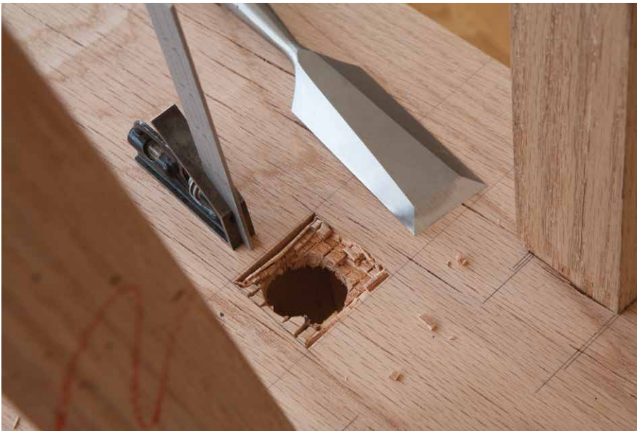
Figure 7.11. All marked up. Here is the underside of the benchtop as I finish the mortise for the planing stop. Lots of pencil lines. Lots of sneaking up on the right dimension. Lots of sharpenings (after each mortise) ensures the walls are crisp.
